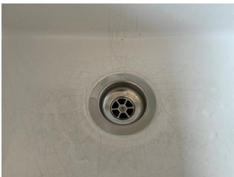
Riss/krakelering i vask.
