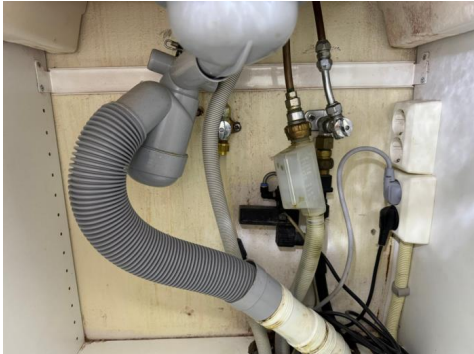
Røropplegg under vask.
