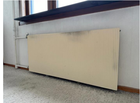
Eldre radiatorovn i stue.
