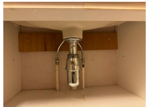
Røropplegg under servant.
