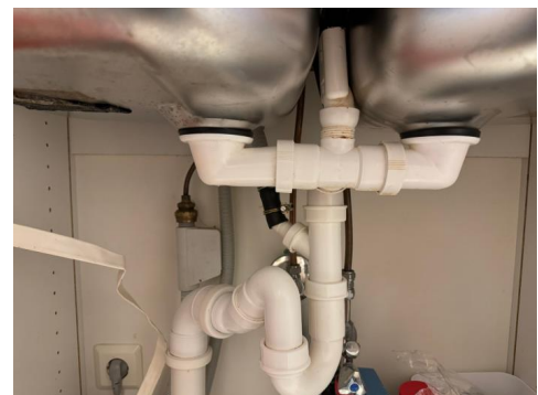
Røropplegg under vask.
