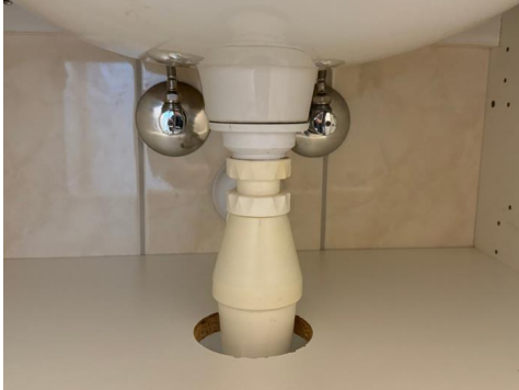
Røropplegg under servant.
