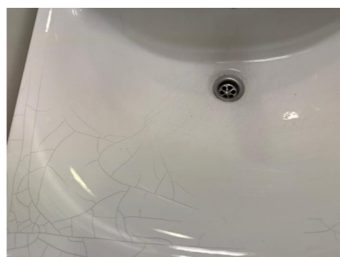
Riss/krakelering i servant.
