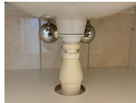
Røropplegg under servant.
